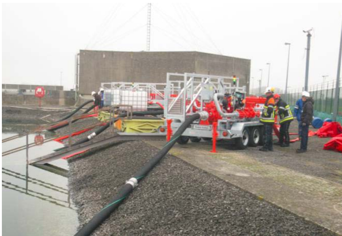
Figure 8: Mobile pumps training at the Doel NPP in the framework of the CSBO strategy.
